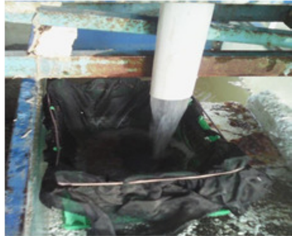
Fig 3: Discharge output tube and diversion sediment and collecting sediment
